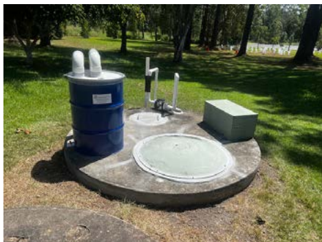
The activated carbon filter atop the septic tank has been hermetically sealed.
